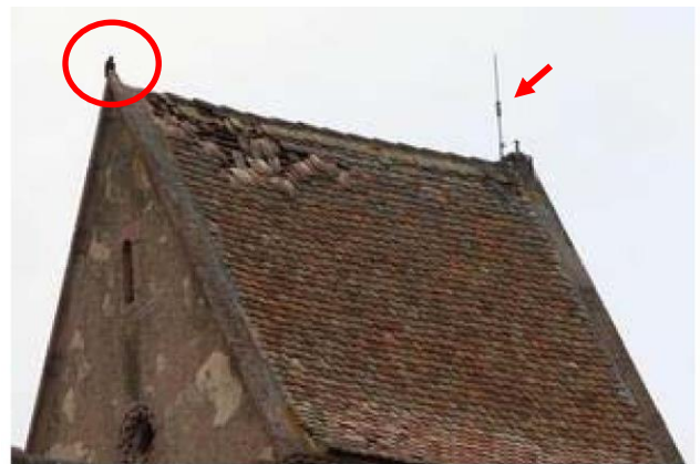
Figure 19. The bell tower showing the remnants of the damaged stone cross (left) and the ESE air terminal (right) about 7 m away. (Picture courtesy of Dernières Nouvelles d'Alsace)
