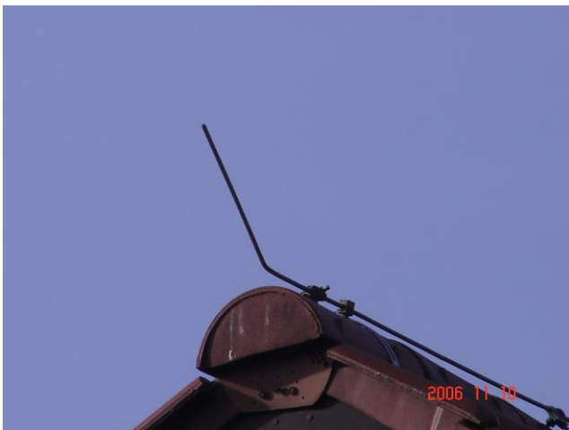
Figure 6. An example of a continuous solid cylindrical conductor applied as an air terminal on the ridge end of the roof.
