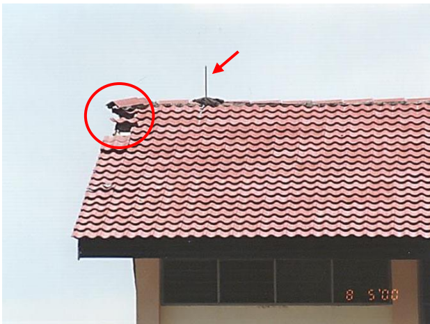
Figure 1. Example of an air terminal (arrowed) incorrectly positioned away from the ridge end of the roof where a bypass (circled) had occurred.
