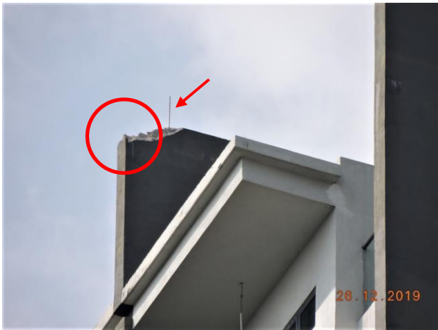
Figure 5. Example of a minor bypass on a roof firewall installed with an air terminal positioned not in accordance with the IEC 62305 standard. If the air terminal had been positioned at the end of the firewall, the bypass could have been prevented.
