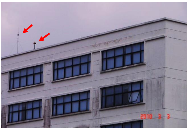
Figure 17. A building photographed with two ESE air terminals.
