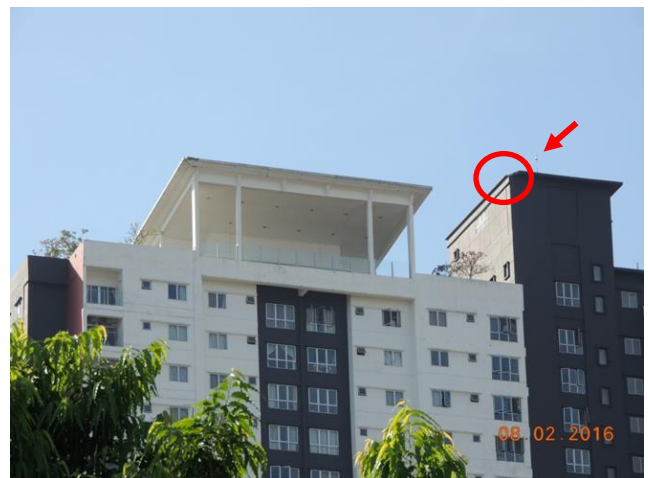
Figure 14. Photograph of the same building with a new bypass taken 5 years later. The old bypass has been repaired.
