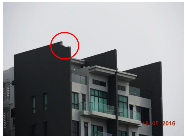
Figure 4. Example of a major bypass on an unprotected part of a roof firewall.
