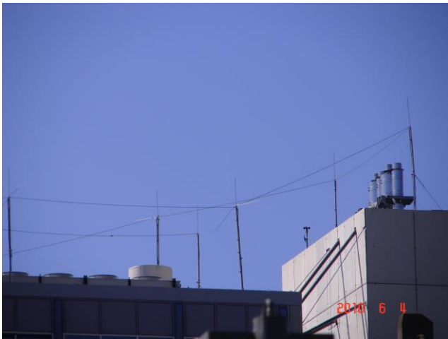
Figure 10. An example of a continuous solid cylindrical conductor suspended high above the roof on masts to protect vulnerable rooftop equipment.
