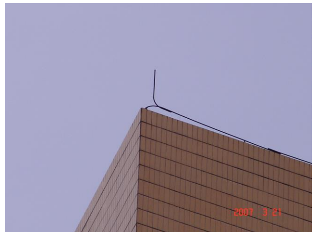
Figure 8. An example of a continuous solid cylindrical conductor applied at the outer corner of the roof.
