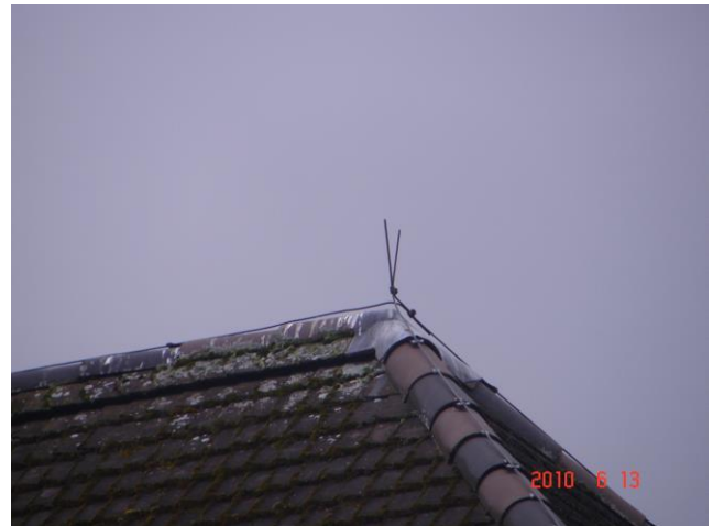
Figure 7. Another example of a continuous solid cylindrical conductor applied as an air terminal on the ridge end of the roof.
