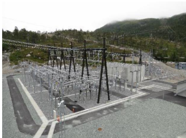
Figure 1. The switching and transformer yard where coupling was evaluated
